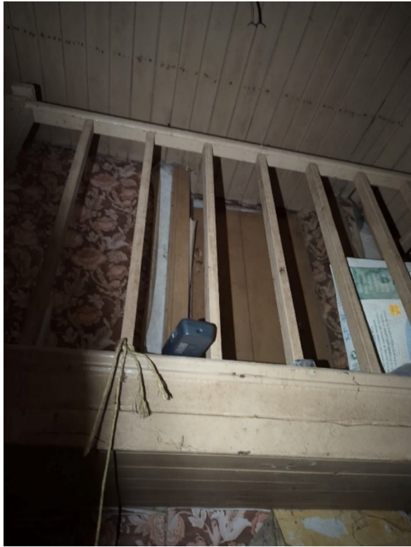
Photograph 36. Door to upstairs loft (Location A, building 2)
