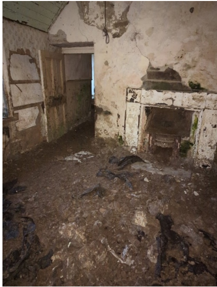
Photograph 34. Location (Location A, building 1) interior in poor state of repair.
