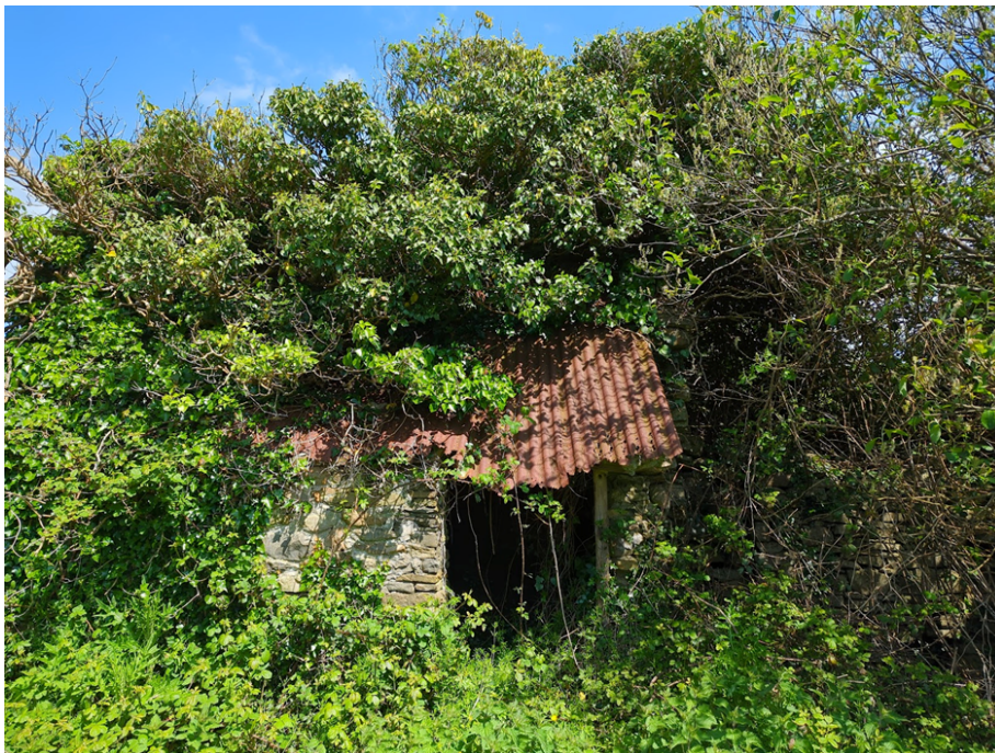
Photograph 39. Old shed in poor state of repair (Location B)
